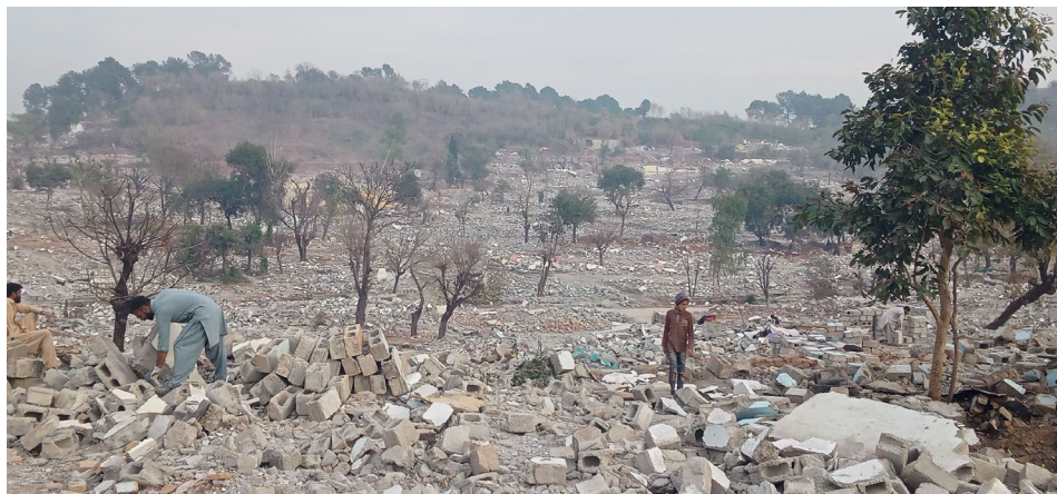
Figure 4. Massive demolitions of informal settlements in Noorpur Shahan
